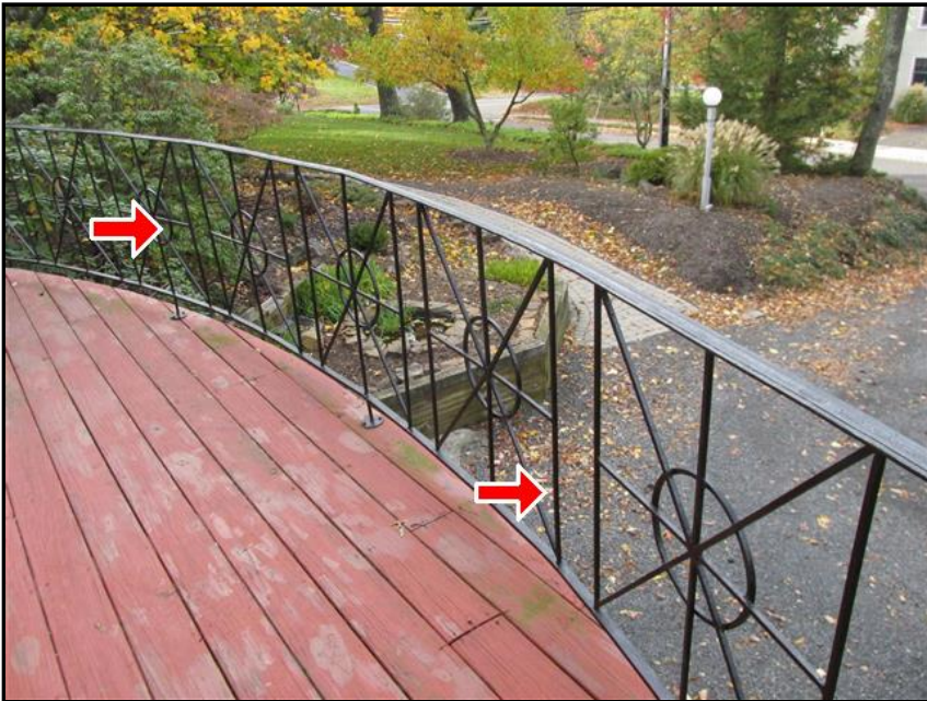
2.3 Item 4(Picture) Balcony railing balusters spaced to far apart.
