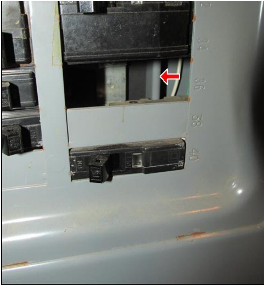
7.1 Item 2(Picture) Missing panel knock out covers.
