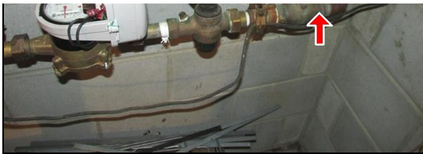
6.3 Item 1(Picture) Main water shut off valve.
