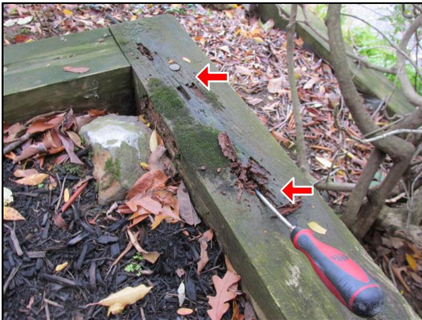
2.4 Item 2(Picture) Damaged timber walls at small areas.
