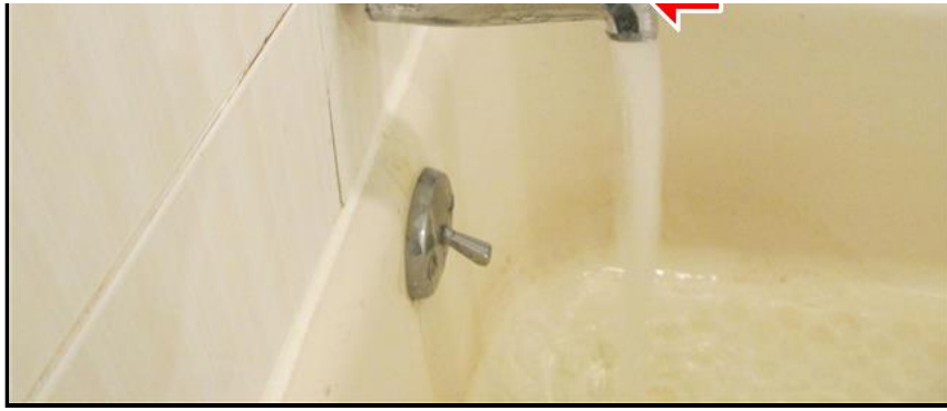
6.1 Item 3(Picture) Spout diverter repairs needed.
