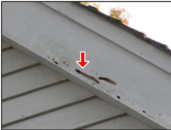
2.5 Item 2(Picture) Damaged fascia boards.
