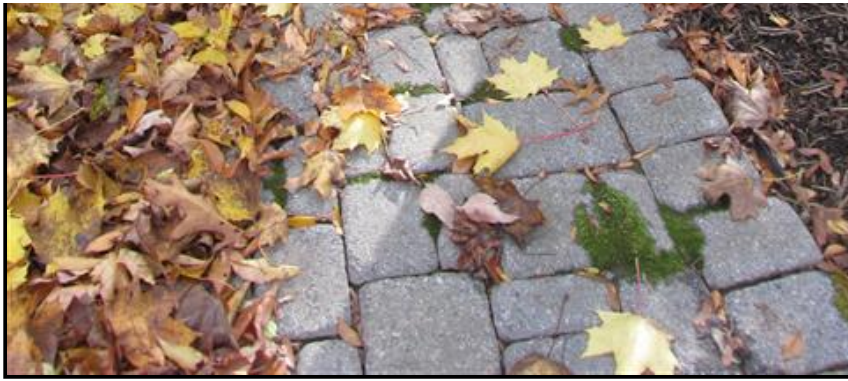
2.4 Item 1(Picture) Walkway erosion occurring.
