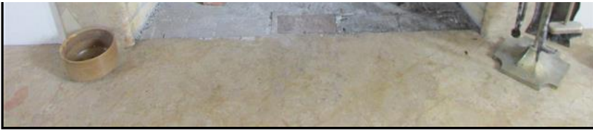
8.5 Item 1(Picture) Chimney sweep needed.
