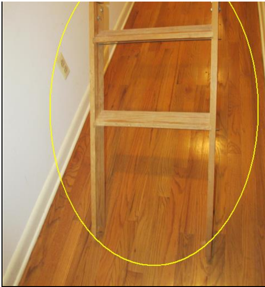
5.5 Item 1(Picture) Attic staircase repairs needed.
