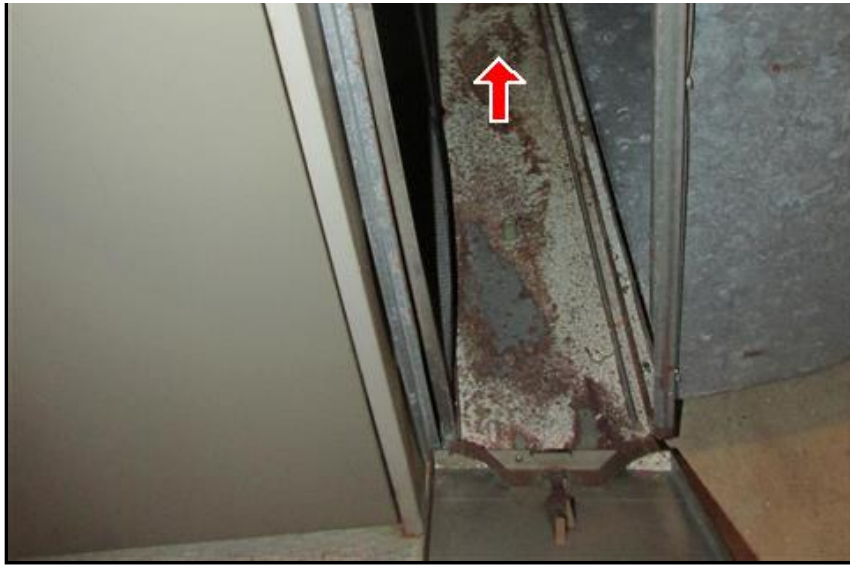
8.3 Item 2(Picture) Missing air filters.
