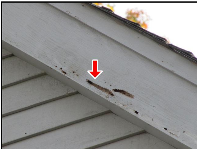
2.5 Item 2(Picture) Damaged fascia boards.
