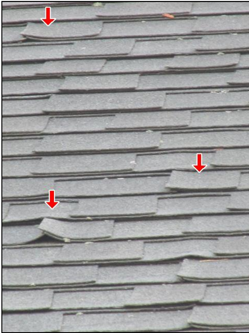
1.0 Item 1(Picture) Aged roofing, repairs / replacement needed.
