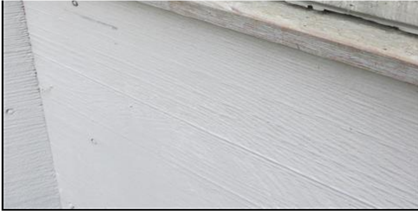
2.0 Item 3(Picture) Lifted siding, loose nail heads.
