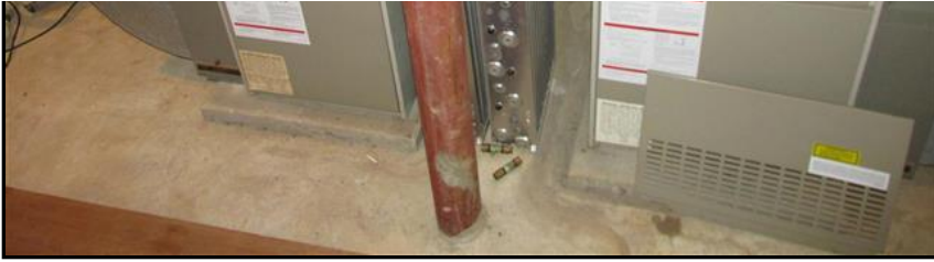
8.0 Item 1(Picture) Aged furnaces.
