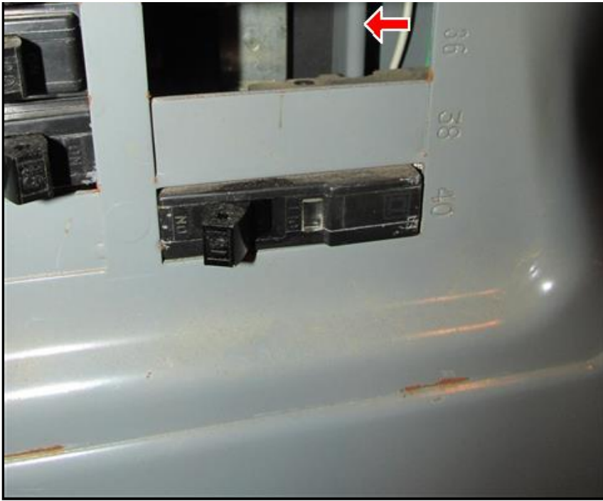
7.1 Item 2(Picture) Missing panel knock out covers.
