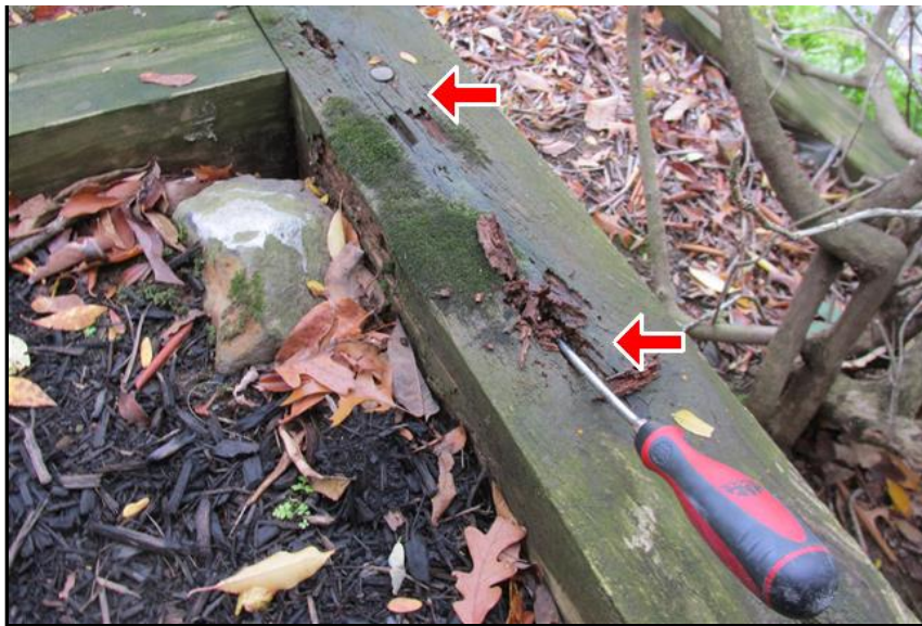
2.4 Item 2(Picture) Damaged timber walls at small areas.
