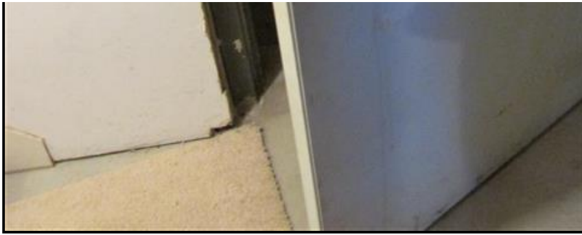
3.4 Item 1(Picture) Missing garage door handle hardware.
