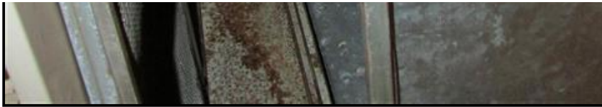
8.3 Item 1(Picture) Open wiring at removed electric air cleaner.
