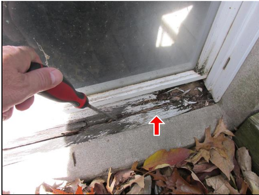
2.2 Item 1(Picture) Deteriorated basement window frame.
