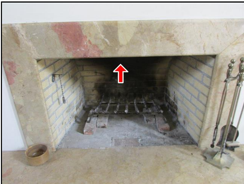
8.5 Item 1(Picture) Chimney sweep needed.
