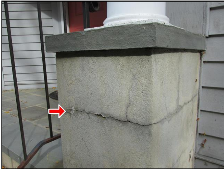
2.3 Item 1(Picture) Porch mortar repairs needed.
