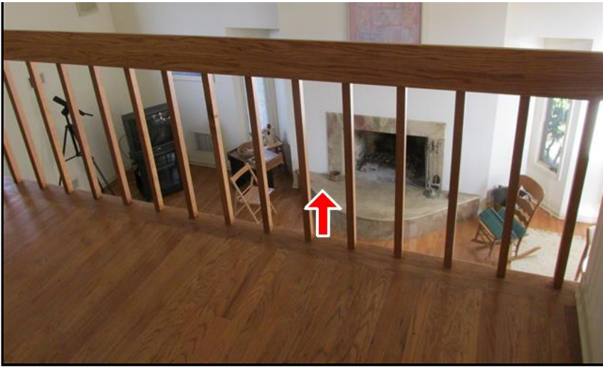
4.3 Item 1(Picture) Spindles spaced to far apart.
