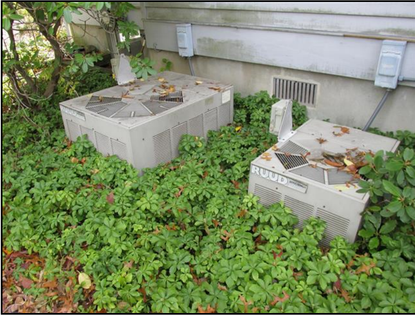
8.8 Item 1(Picture) Aged A/C units. Not tested.
