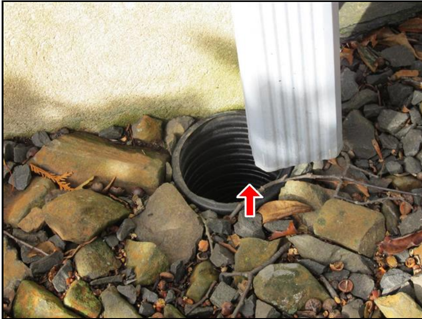
1.3 Item 2(Picture) Downspout connection repairs needed.
