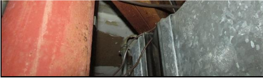
7.3 Item 4(Picture) Missing cover plates.
