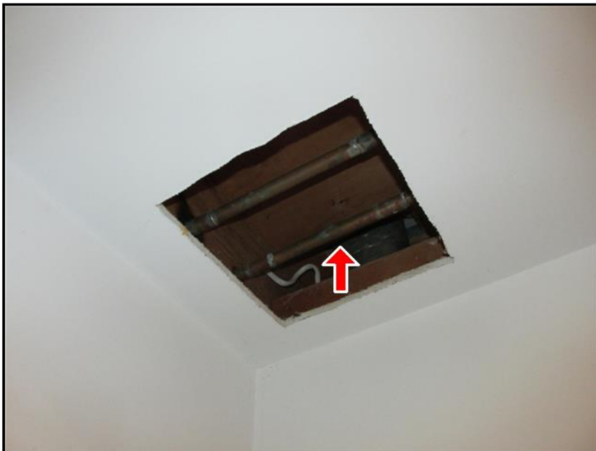
4.0 Item 1(Picture) Ceiling sheetrock repair needed.
