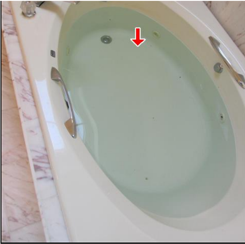
6.1 Item 4(Picture) Jet tub did not function when tested.
