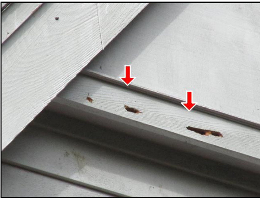
2.0 Item 2(Picture) Damaged trim work.
