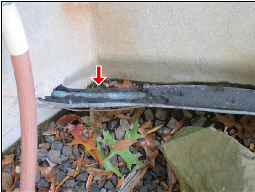
8.8 Item 2(Picture) A/C suction line needs insulation sleeve.
