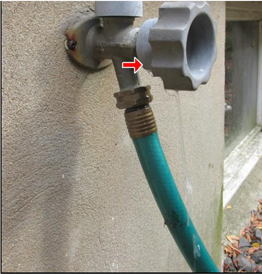
6.1 Item 1(Picture) Hose bib handle leaks.
