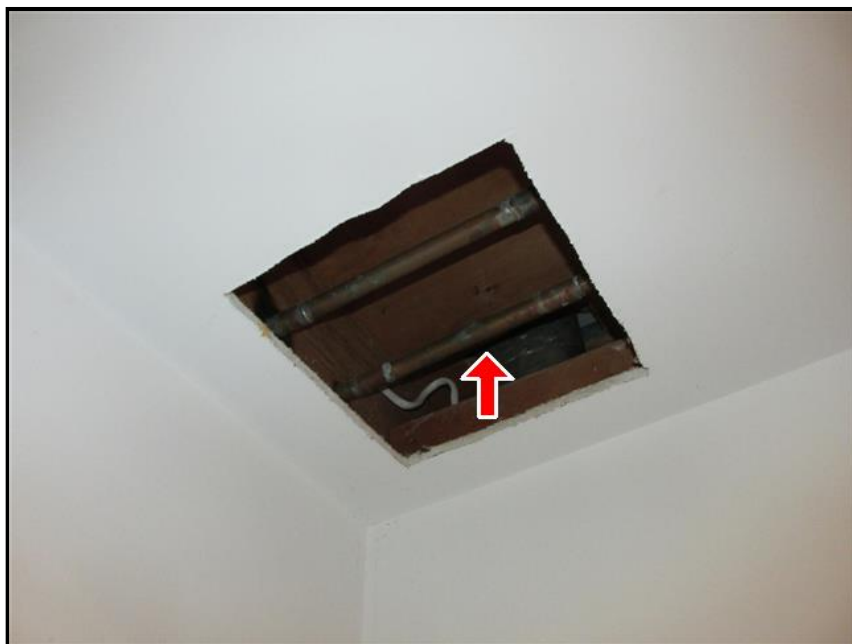
4.0 Item 1(Picture) Ceiling sheetrock repair needed.
