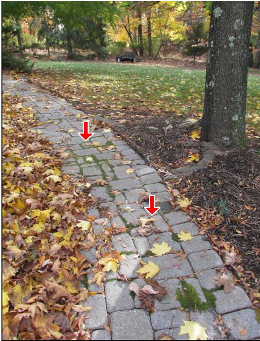
2.4 Item 1(Picture) Walkway erosion occurring.
