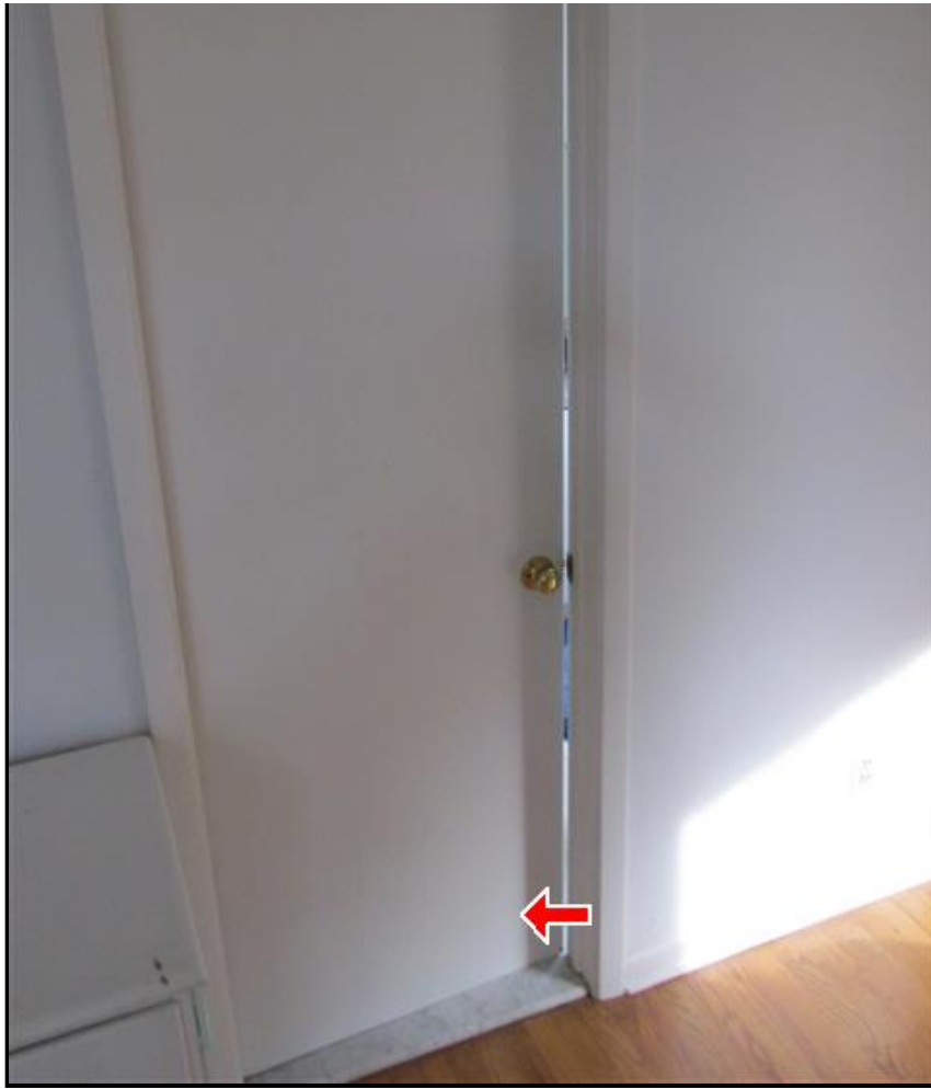
4.5 Item 1(Picture) Bath door repair needed.
