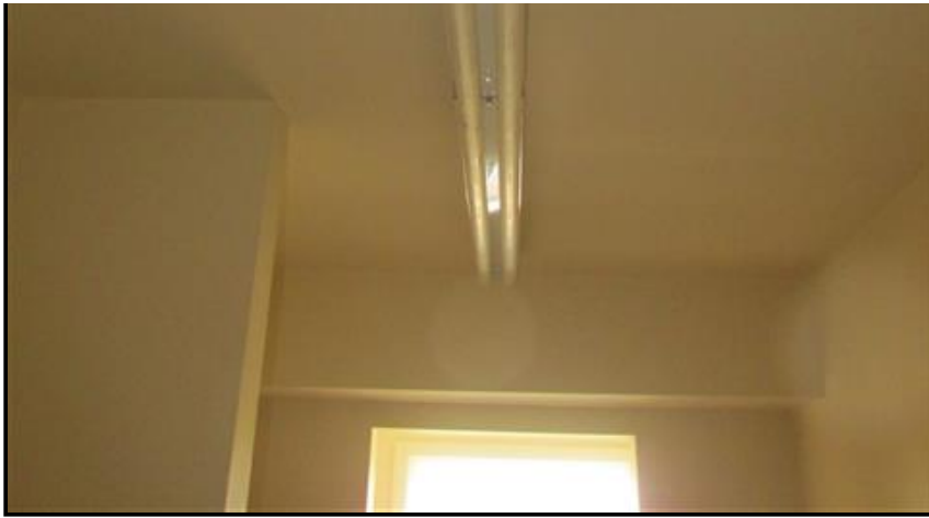
7.3 Item 1(Picture) Noisy light fixture ballast.
