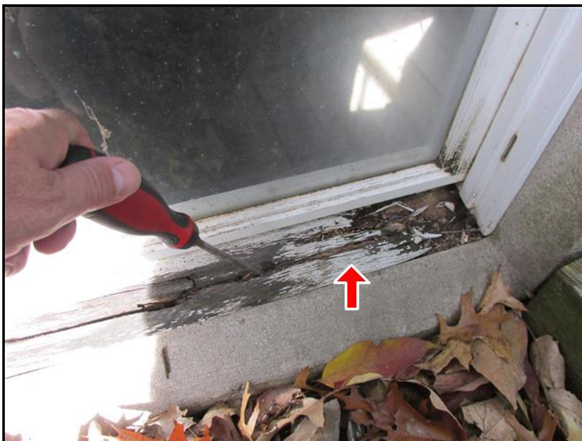
2.2 Item 1(Picture) Deteriorated basement window frame.
