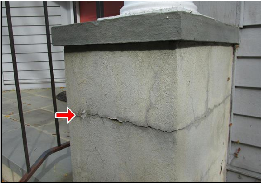
2.3 Item 1(Picture) Porch mortar repairs needed.
