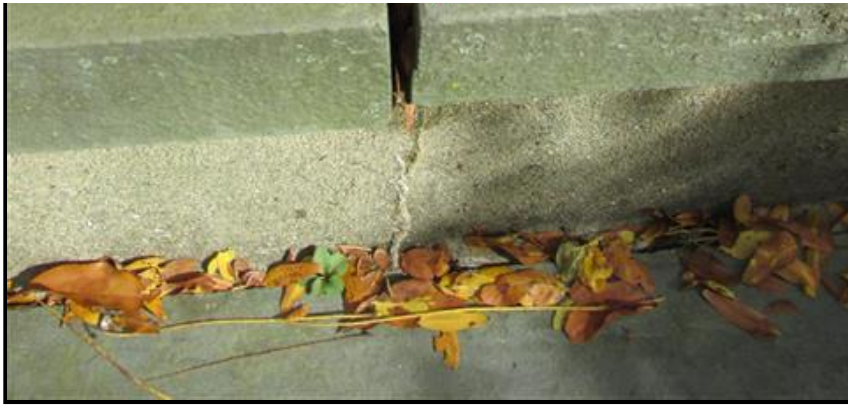
2.3 Item 2(Picture) Porch mortar repairs needed.
