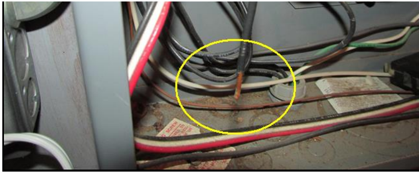
7.1 Item 1(Picture) Open wiring inside electrical panel.
