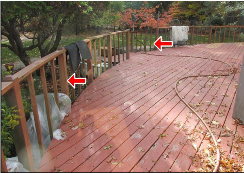
2.3 Item 3(Picture) Deck spindles spaced to far apart.
