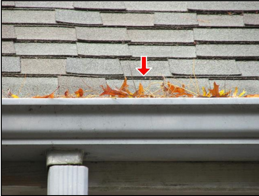
1.3 Item 1(Picture) Gutters need cleaning.
