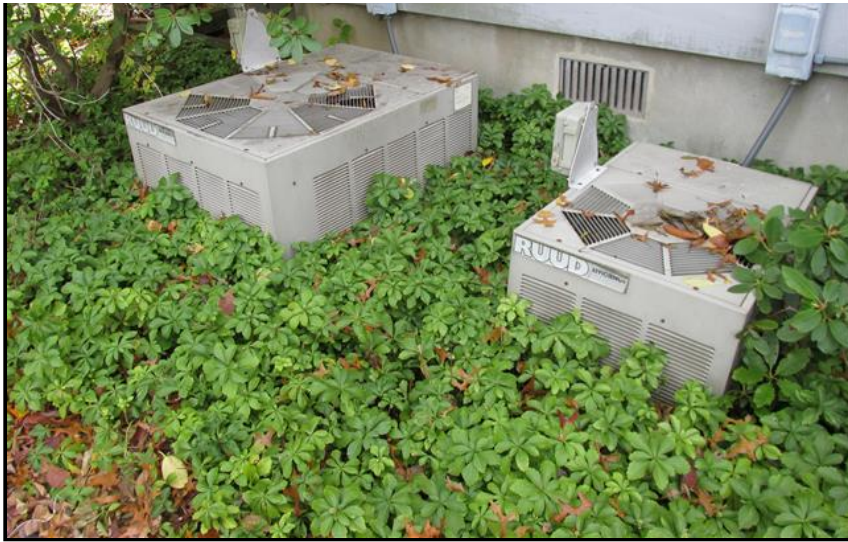
8.8 Item 1(Picture) Aged A/C units. Not tested.
