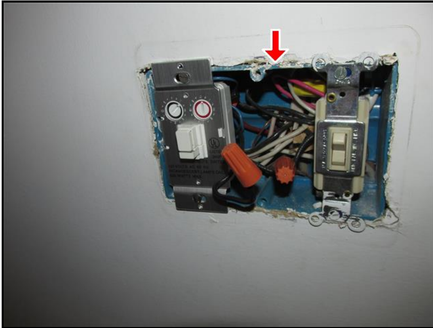
7.3 Item 3(Picture) Missing cover plates.
