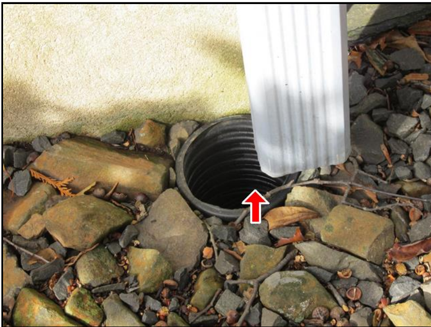
1.3 Item 2(Picture) Downspout connection repairs needed.
