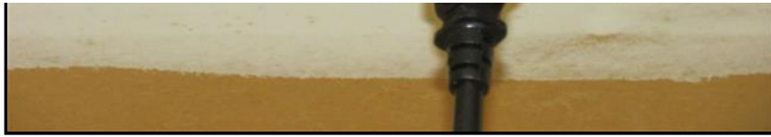
7.3 Item 6(Picture) Amateur light fixture wiring.
