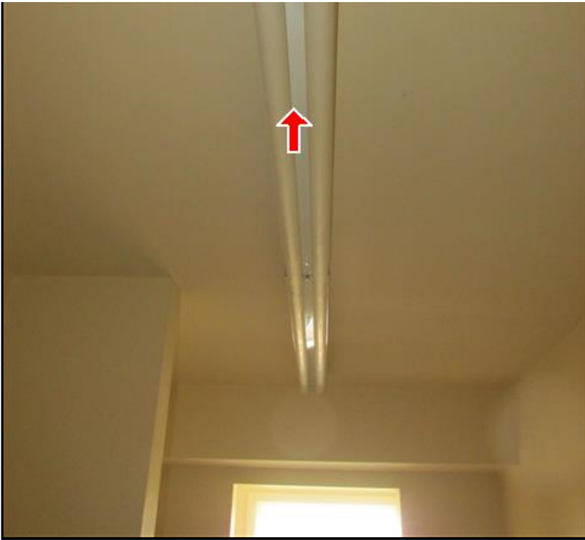
7.3 Item 1(Picture) Noisy light fixture ballast.
