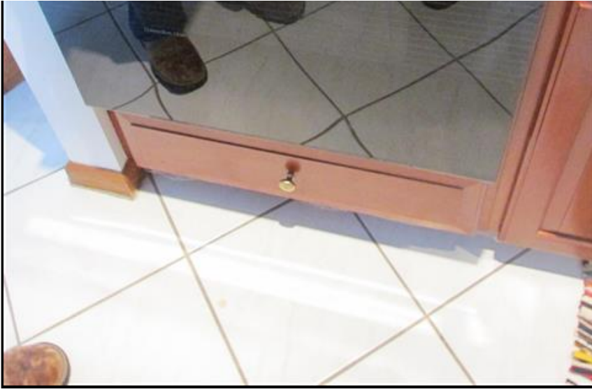
10.1 Item 1(Picture) Oven did not work properly at time of inspection.
