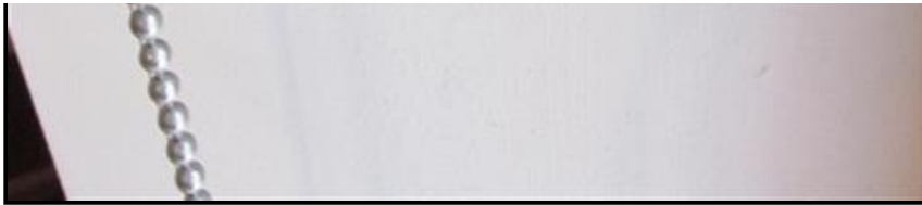
7.3 Item 2(Picture) Missing wall switch.
