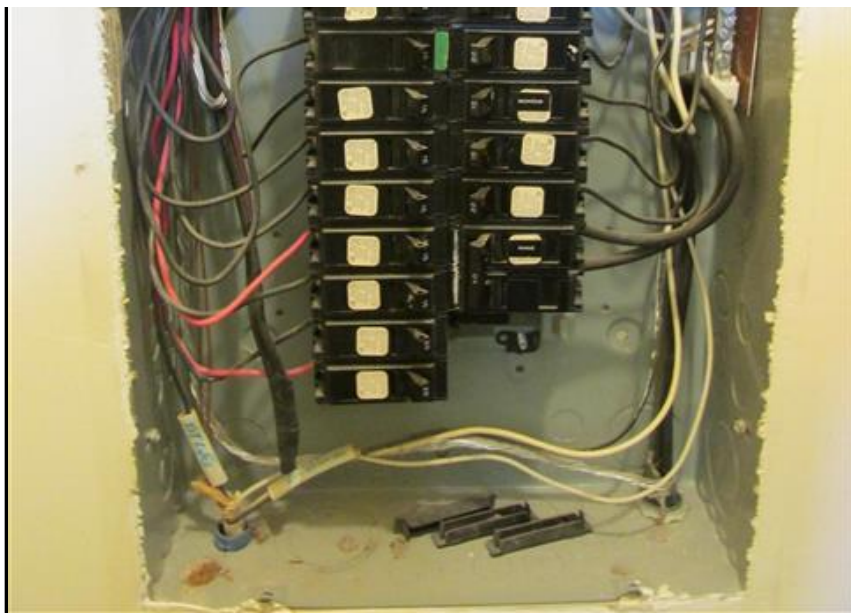
7.6 Item 2(Picture) Sub electrical panel.
