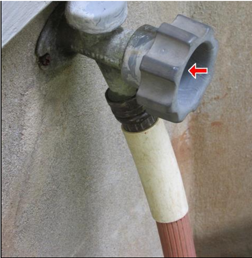
6.1 Item 2(Picture) Hose bib handle damaged.
