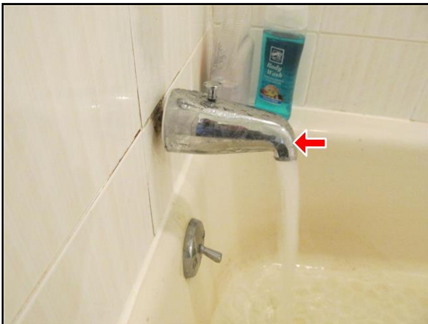
6.1 Item 3(Picture) Spout diverter repairs needed.
