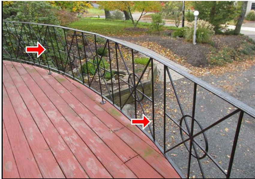
2.3 Item 4(Picture) Balcony railing balusters spaced to far apart.
