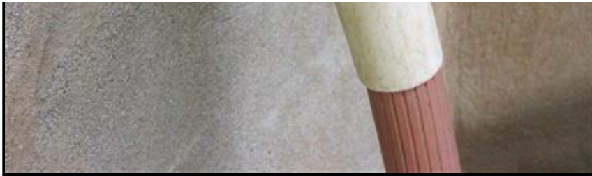
6.1 Item 2(Picture) Hose bib handle damaged.
