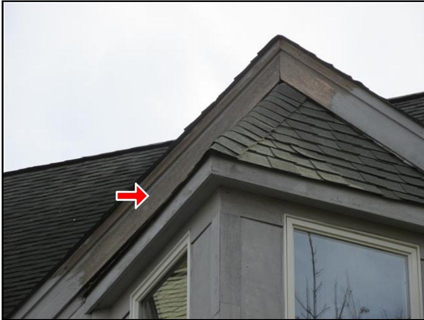
2.5 Item 1(Picture) Prep, prime and paint needed at exterior.
