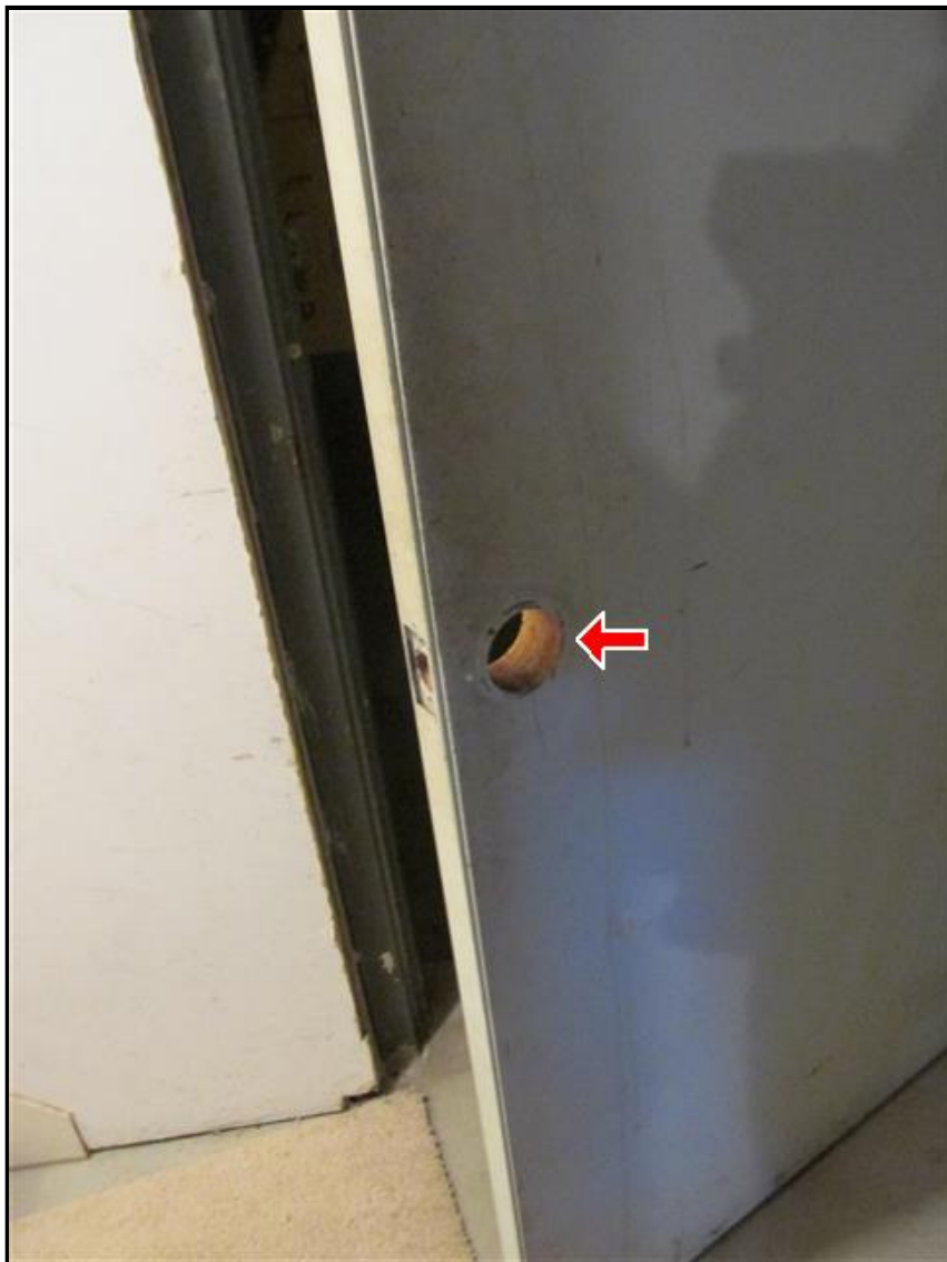
3.4 Item 1(Picture) Missing garage door handle hardware.
