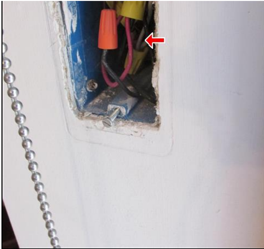
7.3 Item 2(Picture) Missing wall switch.
