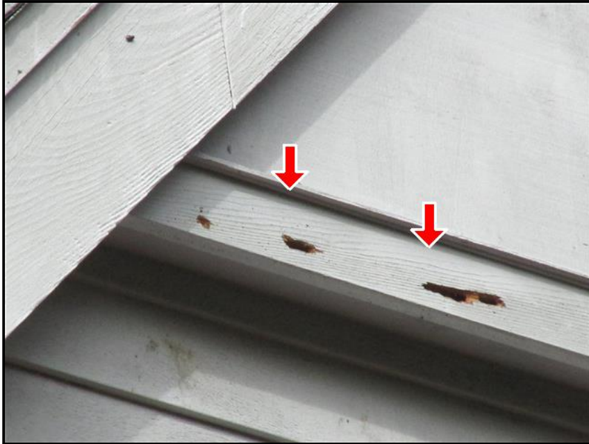
2.0 Item 2(Picture) Damaged trim work.
