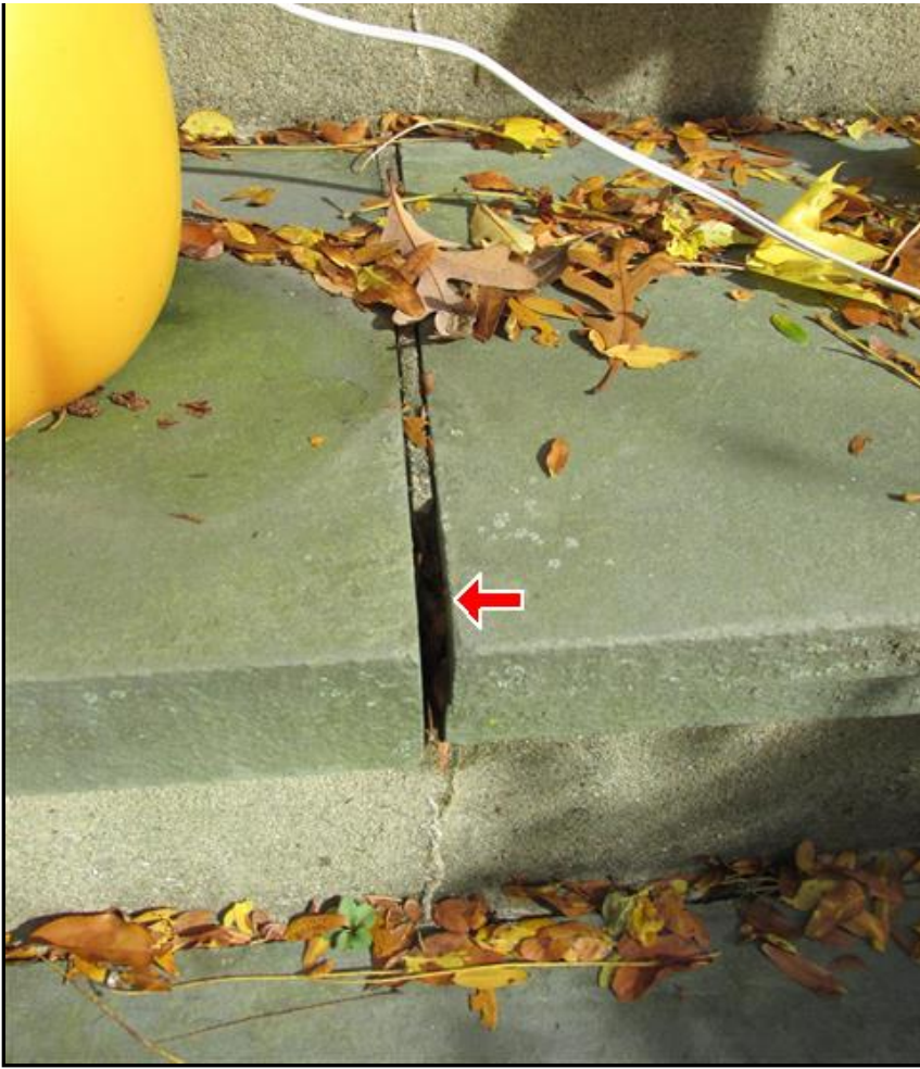
2.3 Item 2(Picture) Porch mortar repairs needed.
