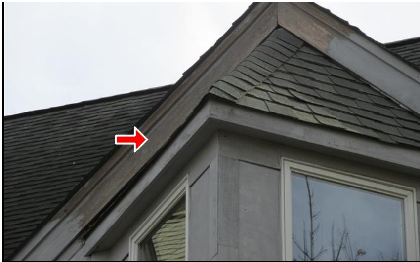
2.5 Item 1(Picture) Prep, prime and paint needed at exterior.
